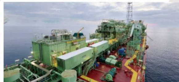
△ Offshore production facility
